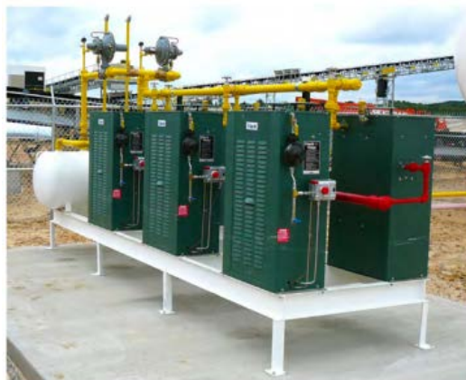
Trailer Mounted Vaporization
